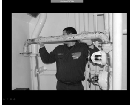
Figure 3. Photo of a “Hard” Bypass 107
