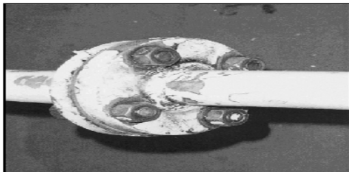
Figure 7. Photo of Worn Flange Bolts 250
