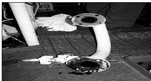
Figure 5. Photo of Sludge inside OWS Discharge Piping 248
