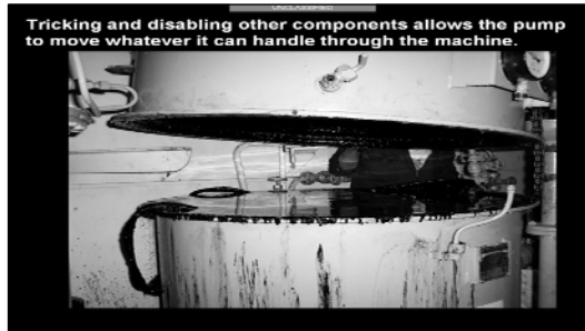
Figure 6. Photo of Sludge Pumped through OWS 249
