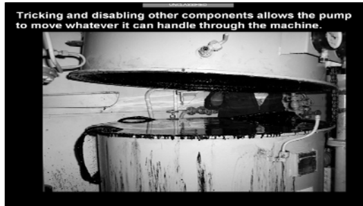
Figure 6. Photo of Sludge Pumped through OWS 249
