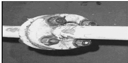
Figure 7. Photo of Worn Flange Bolts 250
